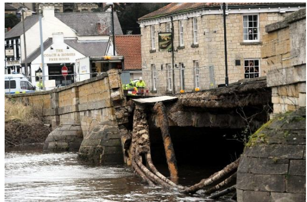
Bridge damage in Tadcaster
