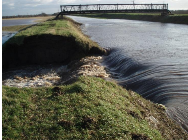
Cheshire Lines flood defence breach near Ormskirk
