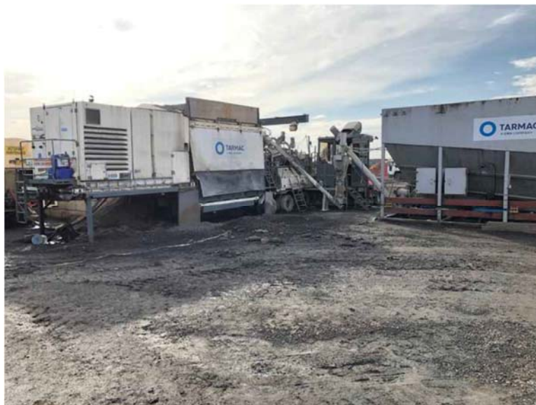
Figure 2. Mobile recycling facility
