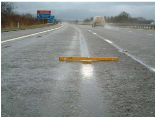
Plate A3.1 Hot Rolled Asphalt (Deformation in Wheeltracks)
