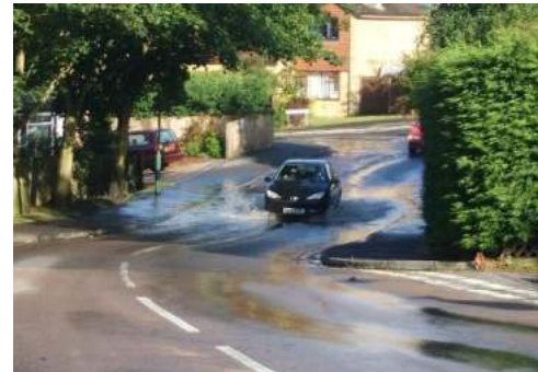
Plate 48b: Inadequate drainage due to root propagation at low point
