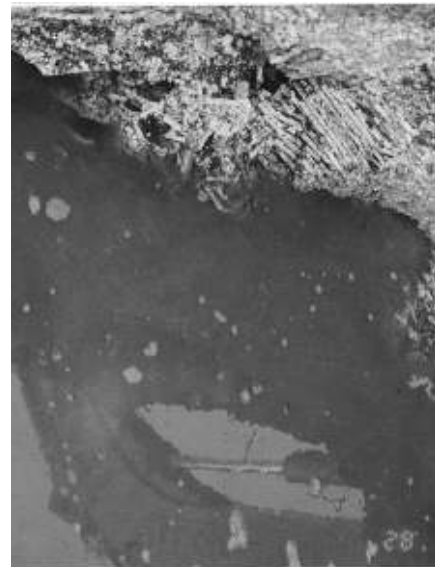
Plate 22b: Road surface showing other run off contamination
