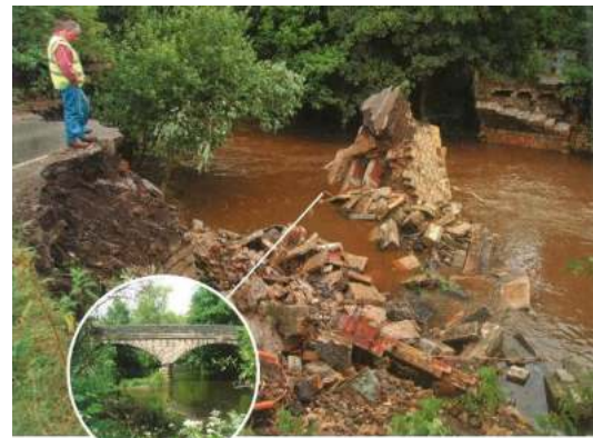
Plate 36: Bridge foundation scour [40]
