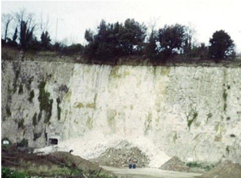
Plate 18: Chalk fall from south facing cliff fall due to local root wedging from crest line trees
