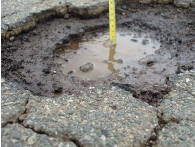
Plate A3.10 Pothole with deterioration of both surface and binder courses. Progressive peripheral deterioration.
