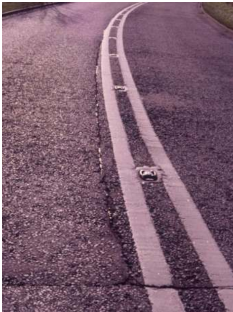
Plate A3.6 Joint located next to lane marking – Not sealed and showing signs of fretting.
