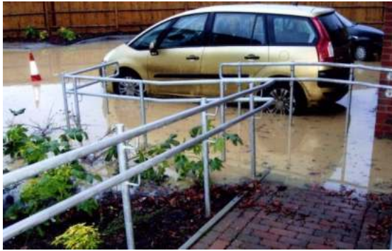
Plate 46: Inadequate capacity of permeable paving
