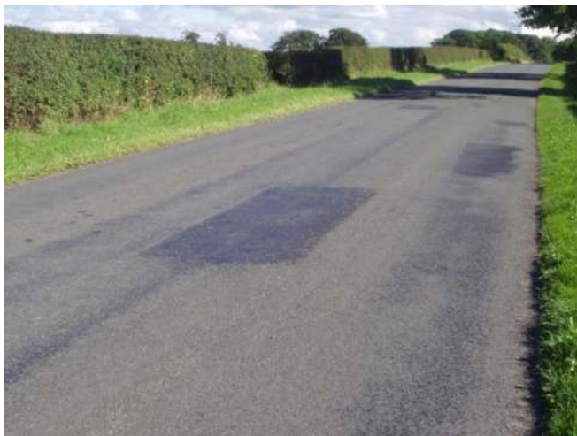
Plate A3.11 Pre-patching with low grade binder asphalt resulting in surface dressing bleeding.
