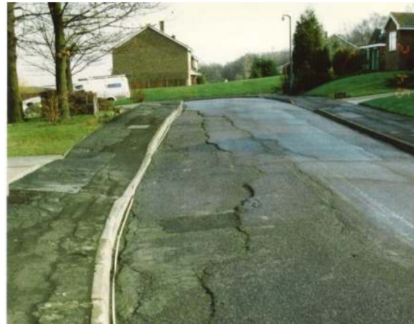
Plate 28: Swelling of clay due to tree removal
