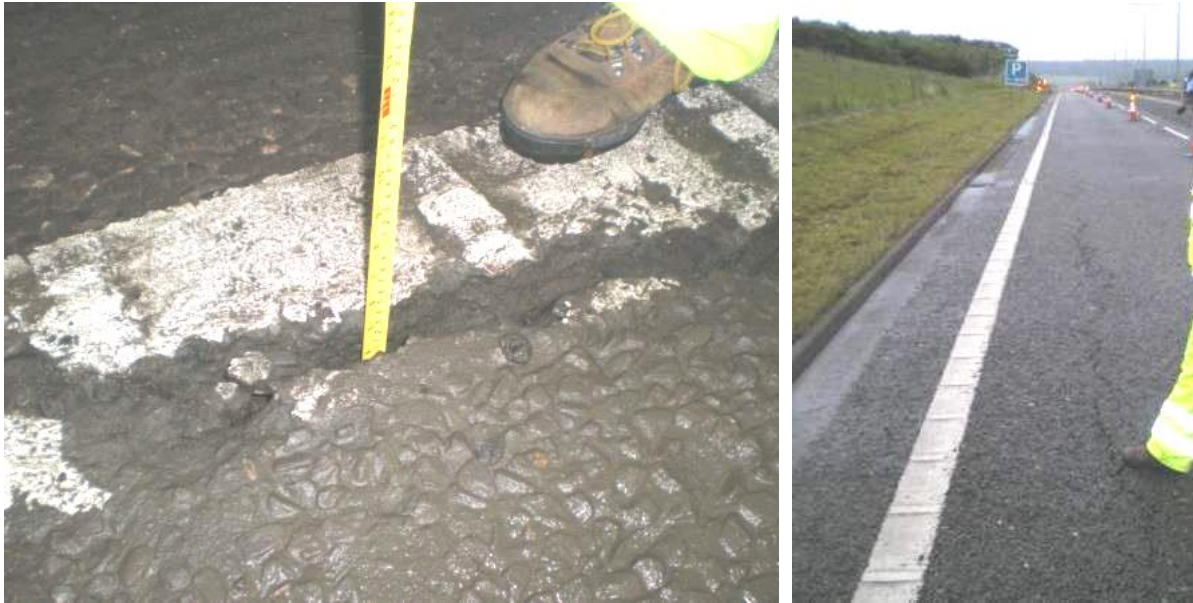
Plates 8 and 9: Carriageway cracking and step on clay soil
