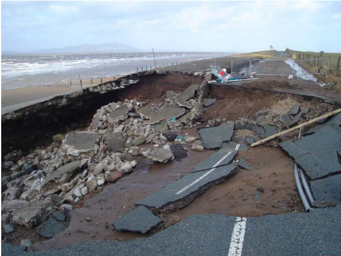
Plate 3.4 B5300 Dubmill Point, Cumbria – collapse due to coastal erosion and inundation from high tides in storm conditions
