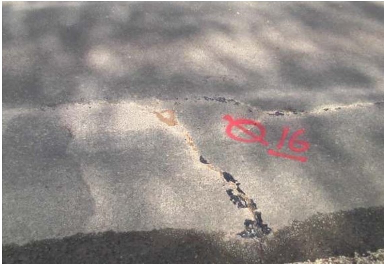
Plate 23: Failure of joint sealants in a concrete carriageway
