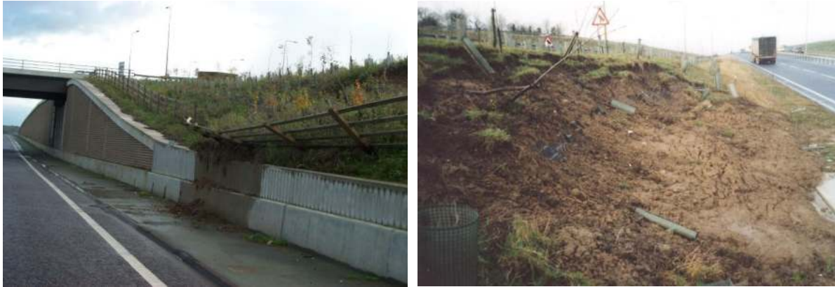
Plates 39 and 40: Shallow slope failure due to surface water run-off from clay slope
