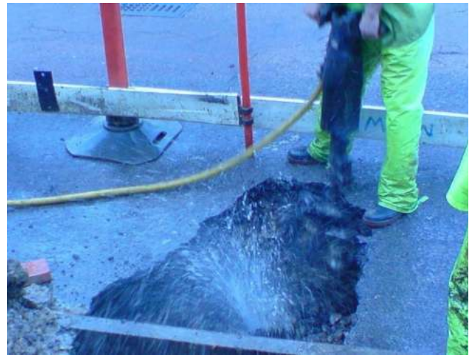
Plate 15: Mains/drains leakage risks increased
