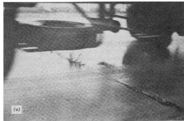
Plate 30: Subgrade pumping of water [36]
