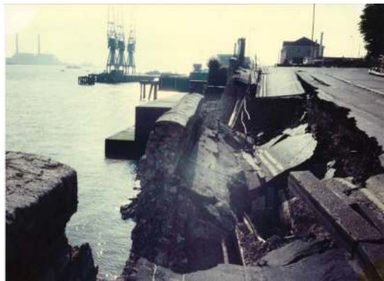
Plate 35: Scour at toe of retaining wall
