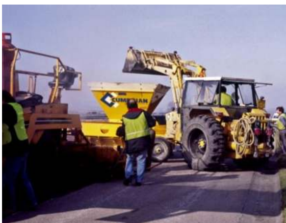
Plates A3.2 & A3.3 Hot rolled asphalt laying process with sufficient access for a tractor to reload the chipper hopper throughout the surfacing process.
