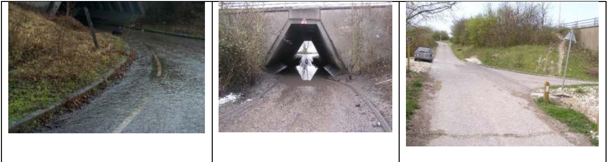
Plates 55: Underpass flooding removed by road ramp
