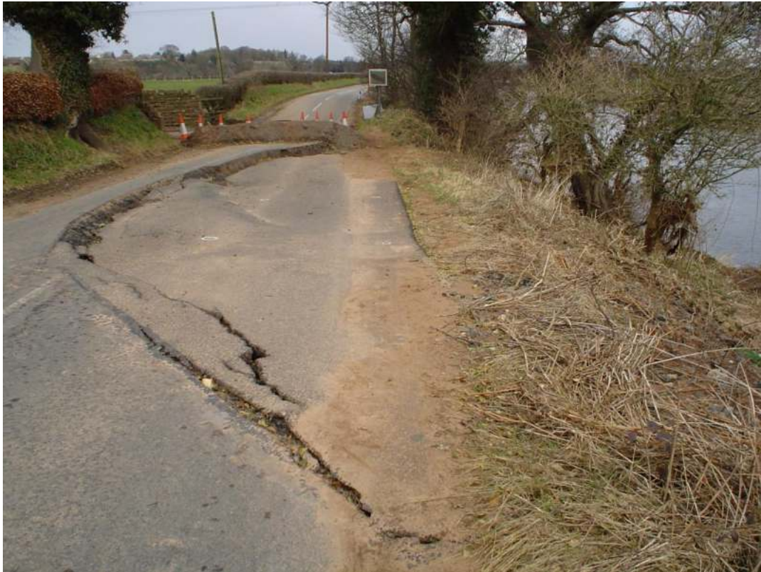
Plate 3.3 Wetheral, Cumbria – toe of slope eroded by the River Eden causing failure after high river levels in January 2006
