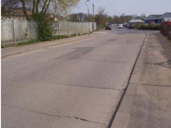
Plate A6.3 Spalling of concrete at edge of joint.
