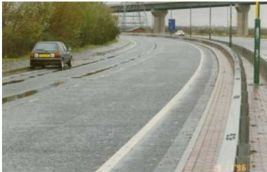
Plate 48a: Inadequate drainage due to surface rutting
