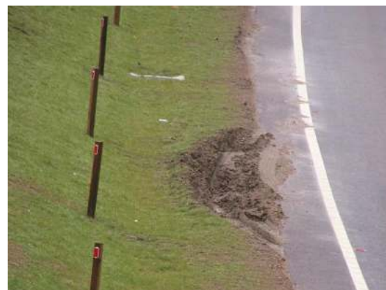
Plate 25: Rutting of softened verge
