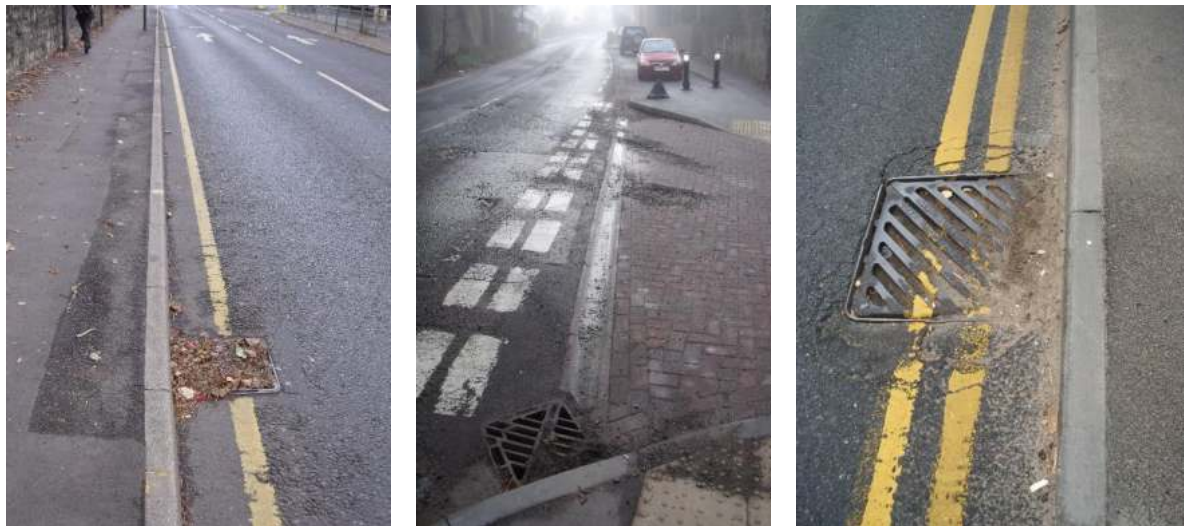
Plates 56: Kerb grate drainage systems
